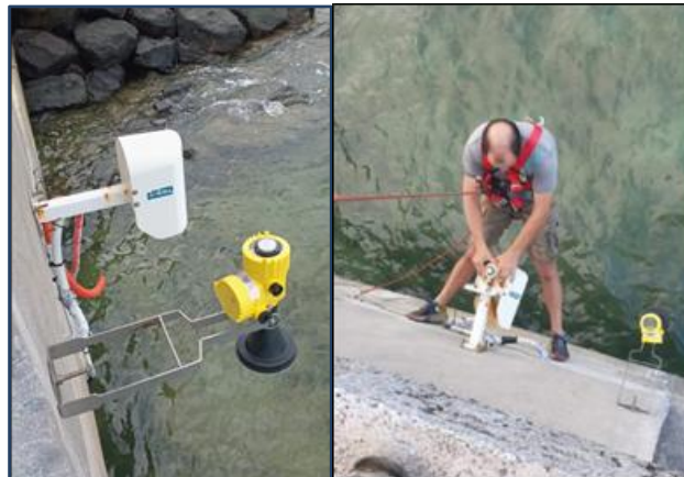
Fig. 30 – Maintenance of the radar sea level station of Wallis.
